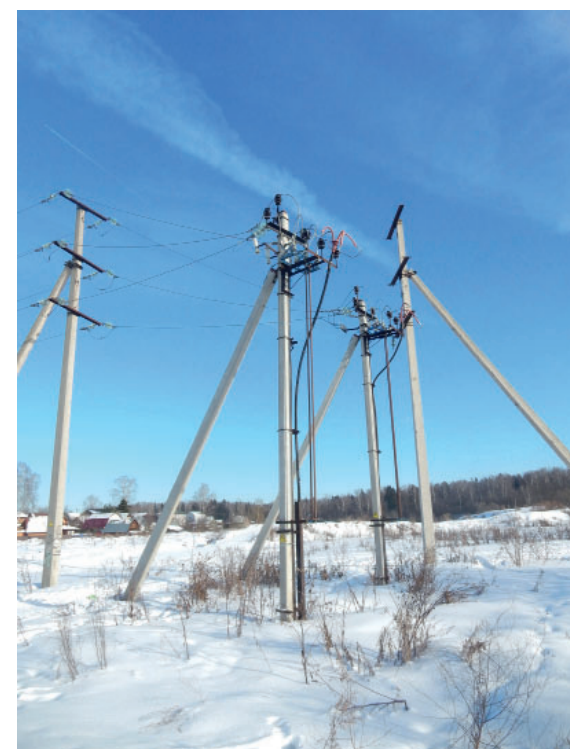
Fig. 1. 10 kV power transmission poles for overhead-underground transition
